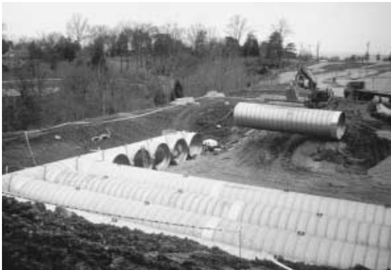
Manifold system used for underground detention.
