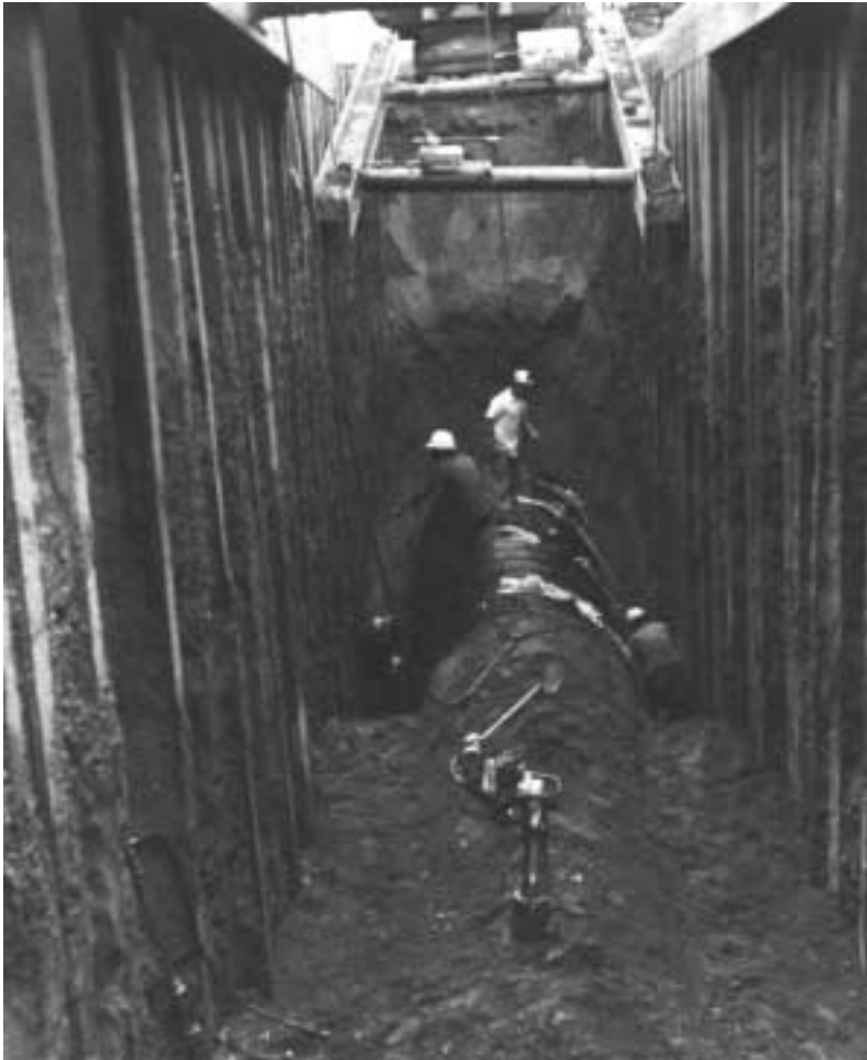
76 mm x 25 mm (3 x 1 in.) full bituminous coated and full paved storm sewer, 820 m (2700 ft), 2200 mm (90 in.) diameter, 1.6 mm (.064 in.).
