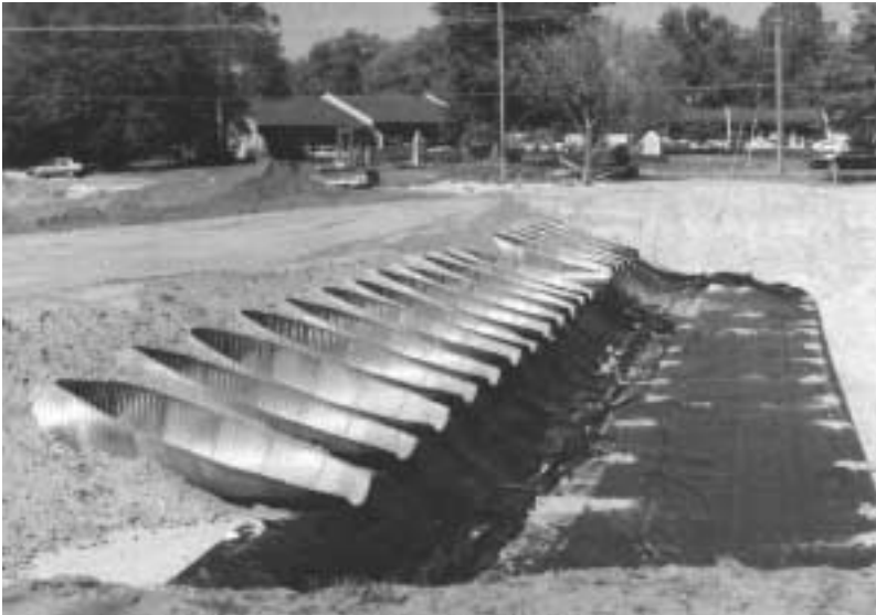
A "Toys R Us" facility in Ocala, FL during construction showing a detention basin constructed of 18 lines of 1200 mm (48 in.) diameter fully perforated corrugated steel pipe used for a recharge system.
