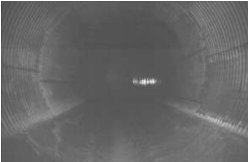
Concrete inverts can solve abrasion problems.
