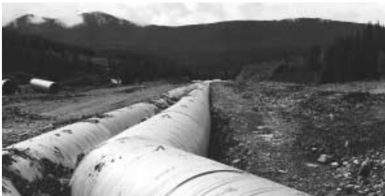
This twin CSP diversion is more than a kilometer long.
