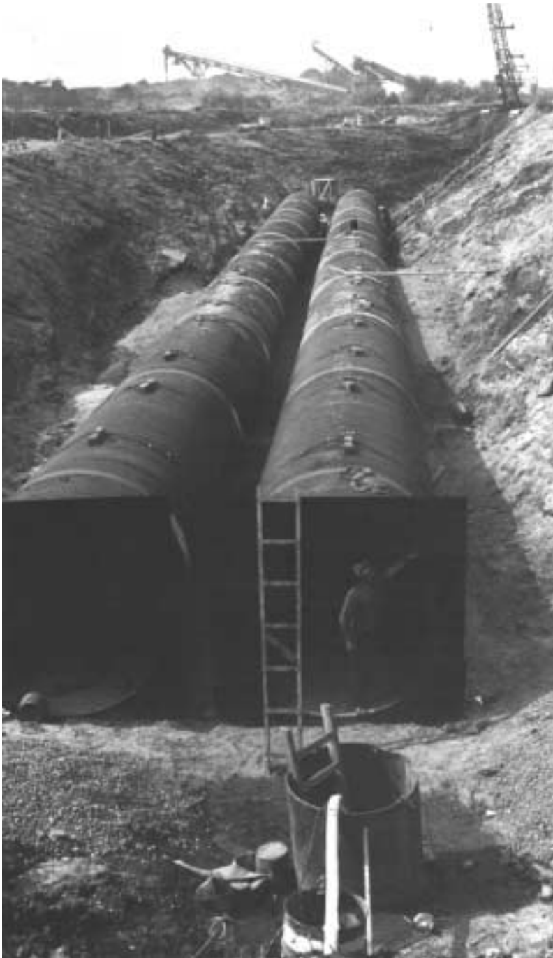
Large diameter structures installed in difficult trench conditions using the advantage of long lengths.
