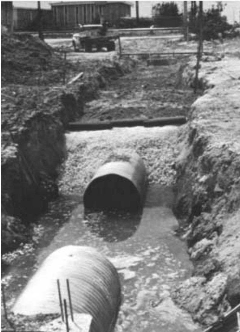
Common recharge trench installation showing relative placement of perforated pipe ballast rock, gravel, and asphalt impregnated building paper.
