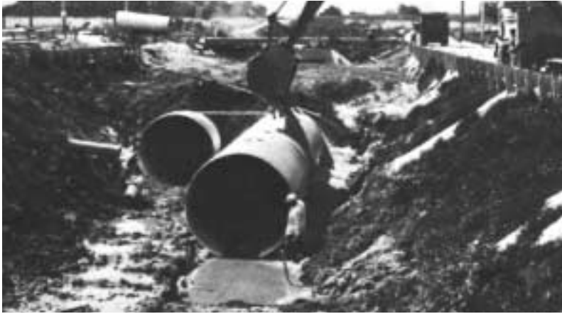
Plain galvanized CSP satisfied service life requirements for storm drains in this environment.
