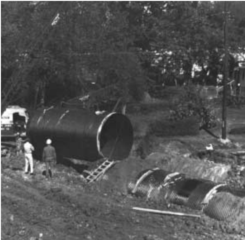
Large diameter twin structures are installed with great savings to the owner.
