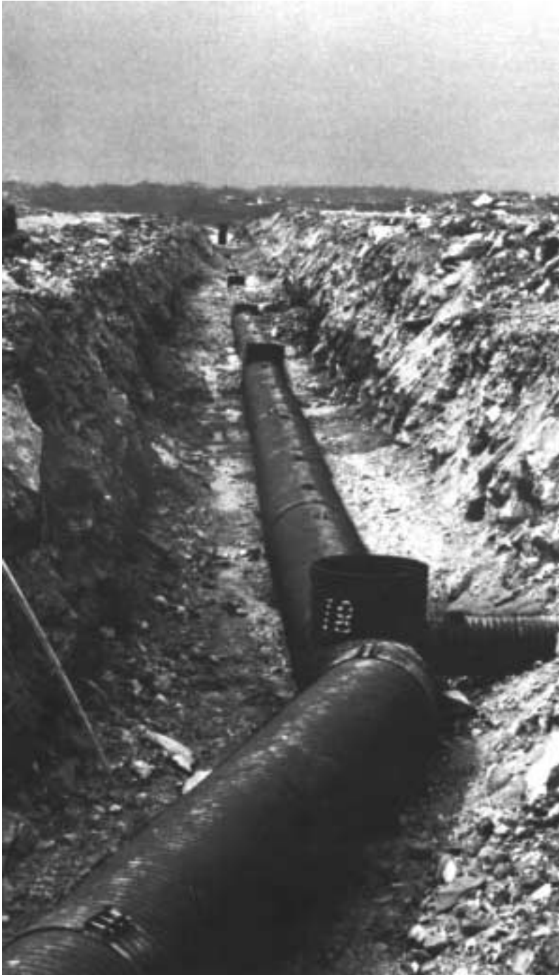
Fabricated fittings reduce head losses in the system.
