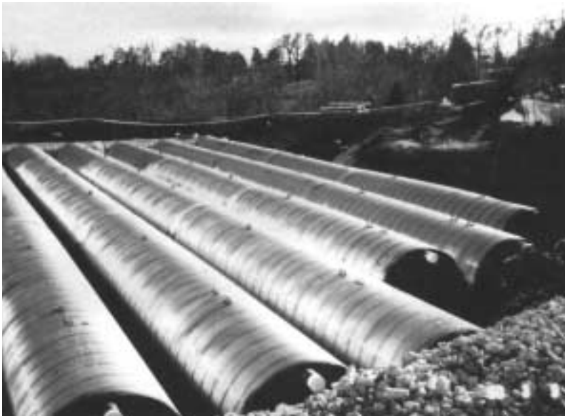
2700 mm (108 in.) diameter CSP used as an underground detention chamber. The outlet control structure is located at the opposite end and to the right of those pipes.
