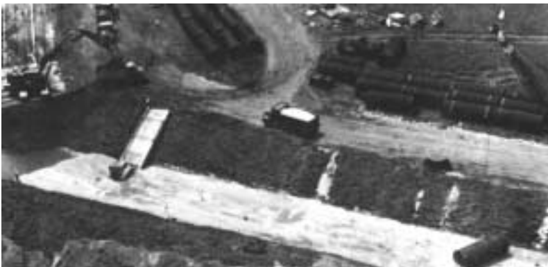
Philadelphia Airport, fiber-bonded, full bituminous coated and full paved CSP with semi-corrugated bands with O-ring gaskets, provides storm drainage for airport— 5800 m (19,000 ft) of 2100 mm (84 in.) through 2550 mm (102 in.) diameters, 2-3 m (6-10 ft) of cover.
