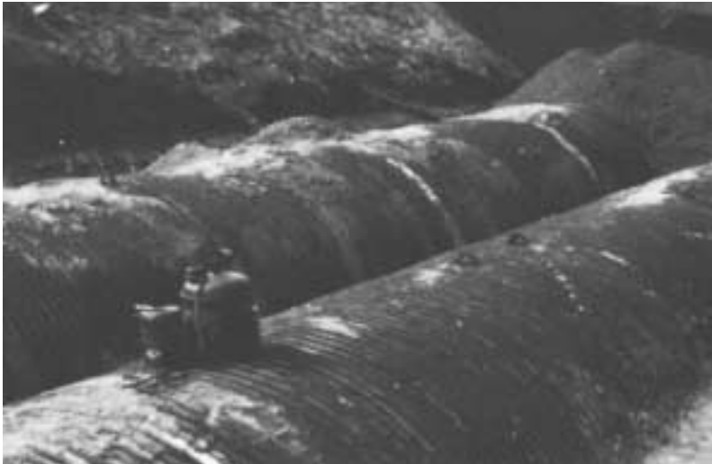
Philadelphia Airport expansion again calls for CSP storm sewers. Corrugated steel pipe was installed 25 years before in an earlier expansion.
