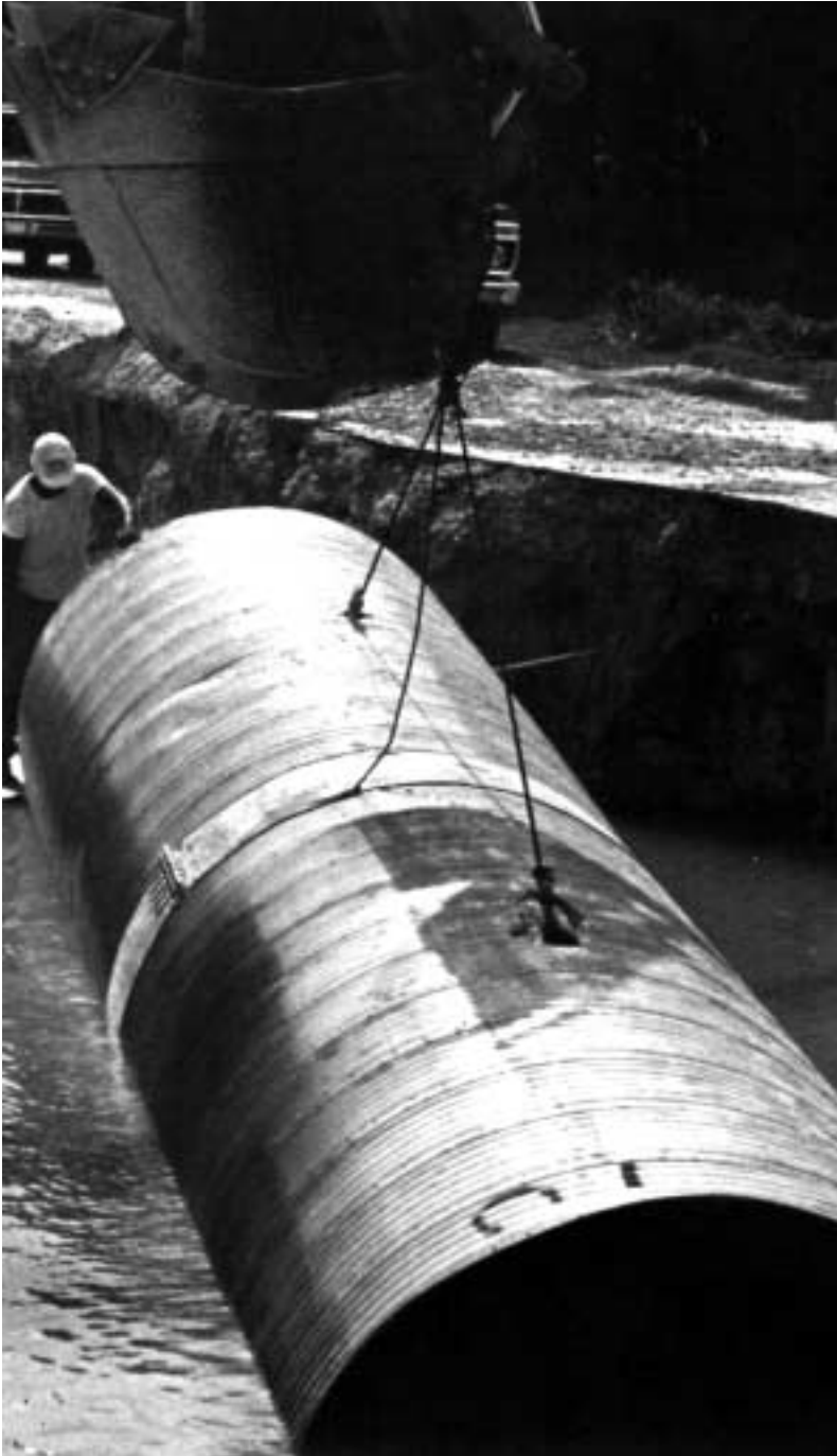
Two 6 m (20 ft) joints of perforated pipe banded together for ease of installation.
