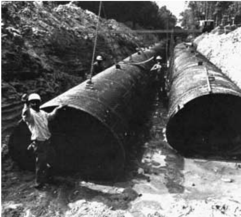
Storm Sewer installation involved 1300 m (4300 ft) of full bituminous coated full paved pipe arch.
