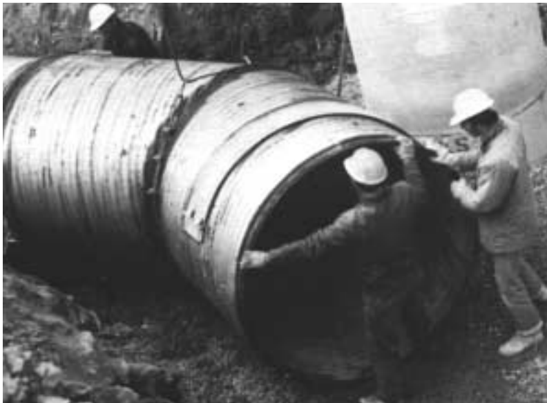
Pre-fabricated miter section of CSP is lowered into place to match bend in trench.
