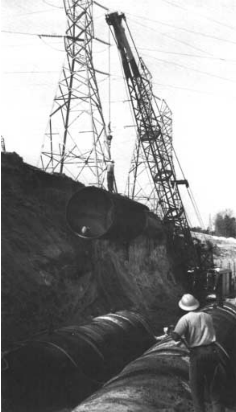
Twin 180 m (590 ft) long smooth line, 2400 mm (96 in.) diameter provide cooling water at the Crist Steam Generating Plant of Gulf Power Company.
