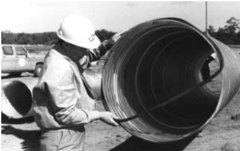
“O-Ring” being placed over the end of the pipe and recessed into the end corrugation.
