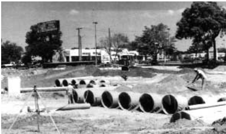
A view of the 18 lines of 1200 mm (48 in.) diameter fully perforated corrugated steel pipe used as a recharge system.
