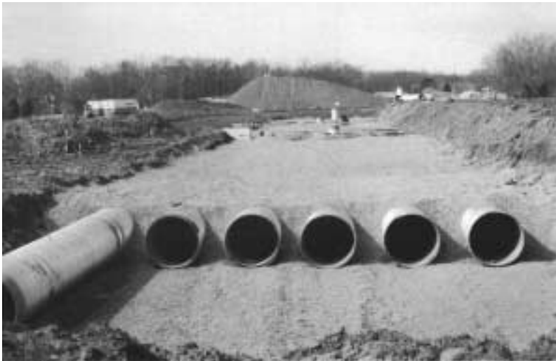
One of two corrugated steel pipe detention chambers constructed on this industrial tract, each consisting of 730 m (2400 ft) of 1200 mm (48 in.) diameter pipe, located in Chantilly Park, VA, a few miles south of Dulles Airport.
