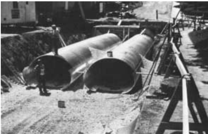
Multiple inline storage installation.
